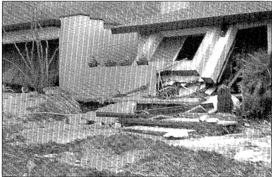
Figure 6. Fast-moving floodwaters caused scour, erosion and structural damage to numerous Rancho Mirage, California homes in September 1976 and in July 1979.
